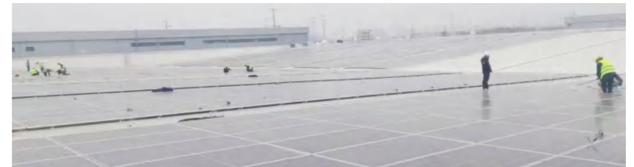
Rooftop Photovoltaic Installation
